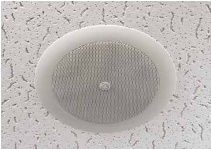
FAP40T (Shown Installed in Drop Tile Ceiling)
